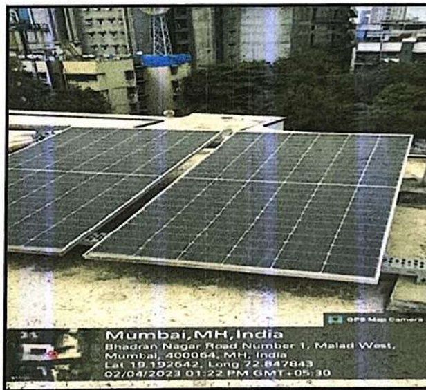
Photograph of Roof Top Solar PV Plant:
