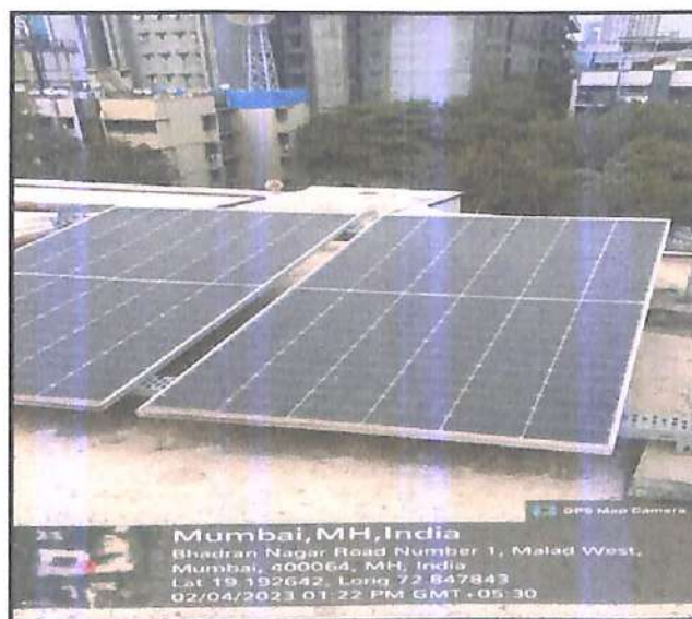
Photograph of Roof Top Solar PV Plant:
